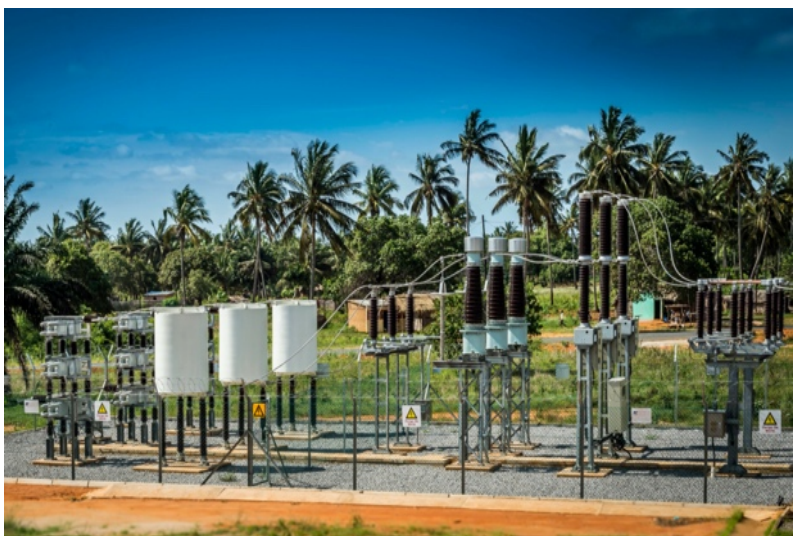
EPC: EdM 110kV Harmonic Filter Bank
