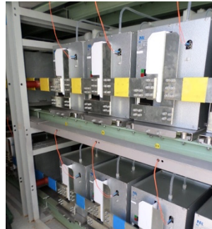
NR Statcom containerised valve
