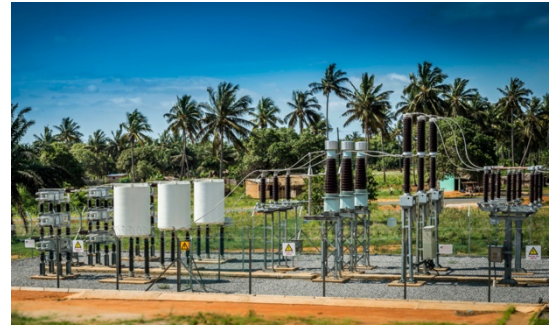
EPC: EDM 6x 110kV Harmonic Filter Banks
