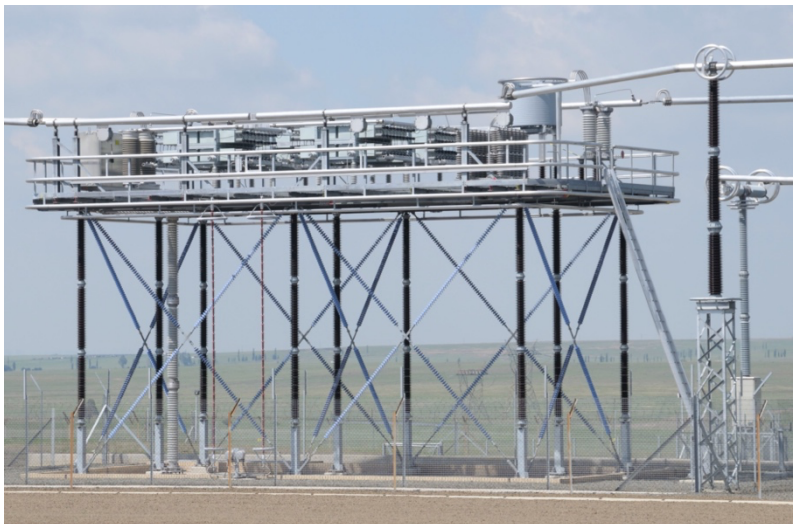
Installation: ABB 3x 765kV Series Compensation
