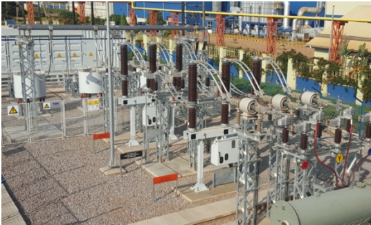
EPC: UMEME 6.6kV ±30MVar Statcom
