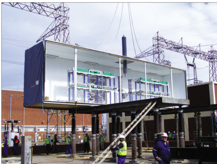
Fig. 4: Capacitor bank in place.
